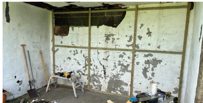
Before: Dunford Road Bus Shelter had seen better days
